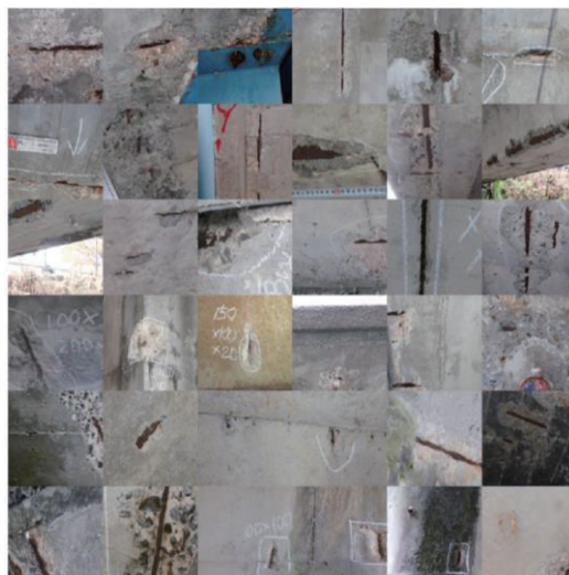
Figure 5: Input images of bridge rebar exposure
