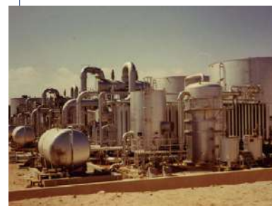
1977 Zliten Seawater Desalination Plants (Libya)
