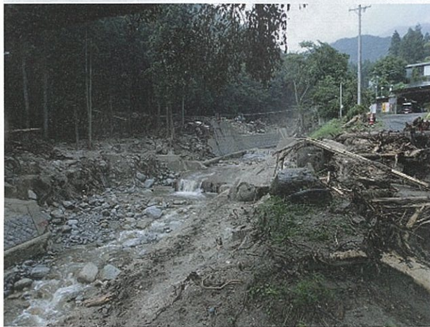
写真-3 流路工の損傷状況 Photo 3 Damage to channel works
