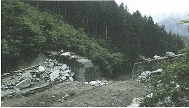
写真-11 梨子沢第1砂防堰堤の堆砂状況 Photo 11 Sedimentation in Nashizawa dai-ichi sabo dam
