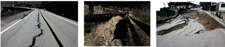
Fig. 9. Crack and stratum color segmentation K-means clustering results.
