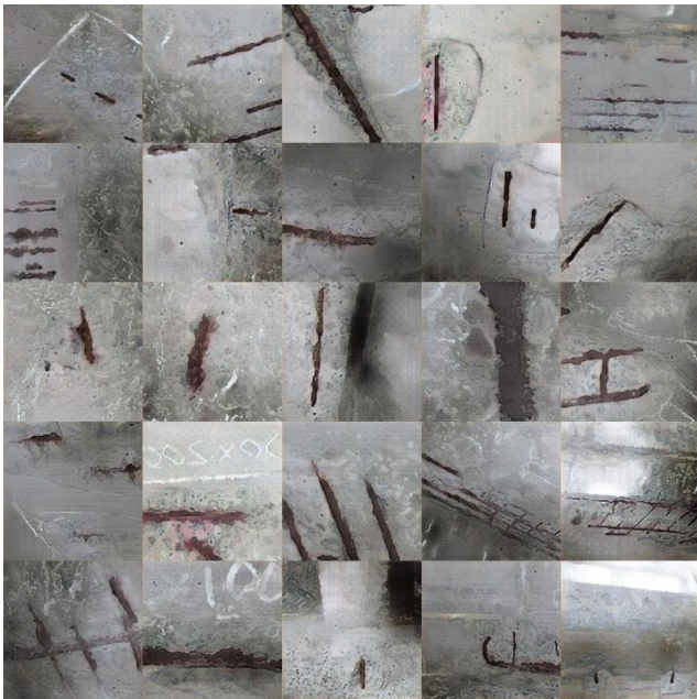
Figure 2: Generated images using synthetic augmentation using L1-Conditional GAN in case of rebar exposure at concrete bridge.
